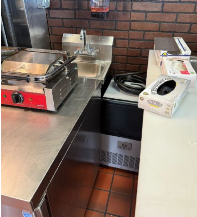
March 13, 2025: Blocked handwashing sink.
