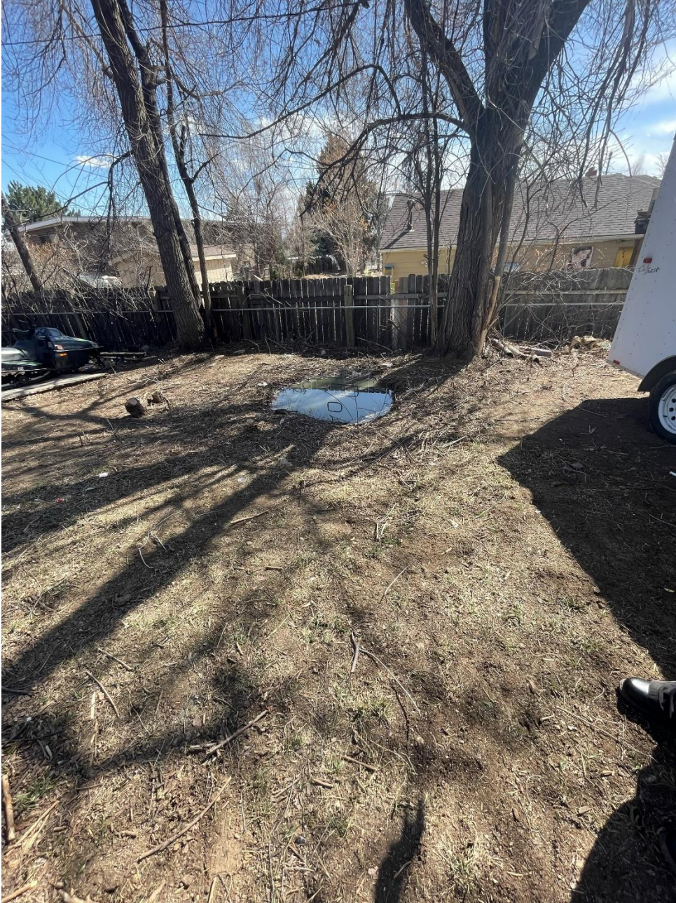
Full scale photo of standing effluent, showing neighboring fence line directly behind the tank (South)
