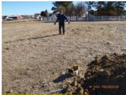
Diverter valve to STA 2 facing east
