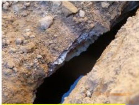
Hole at outlet access port – secondary tank
