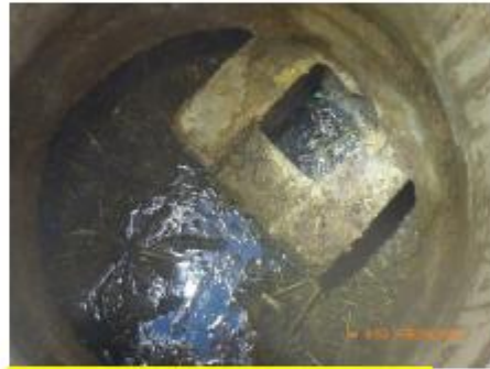
Outlet access port opening – primary tank
