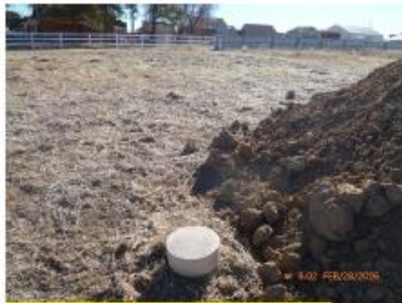
Diverter valve to STA 1 facing southeast
