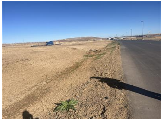
10. Culvert and road base approach needed at access from Quincy Ave to ROW between STR 688 and 687. View facing E.
