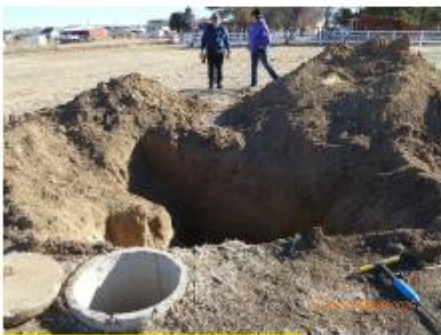
Tank to diverter valve facing east
