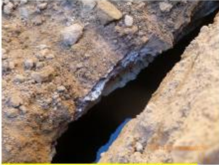
Hole at outlet access port – secondary tank
