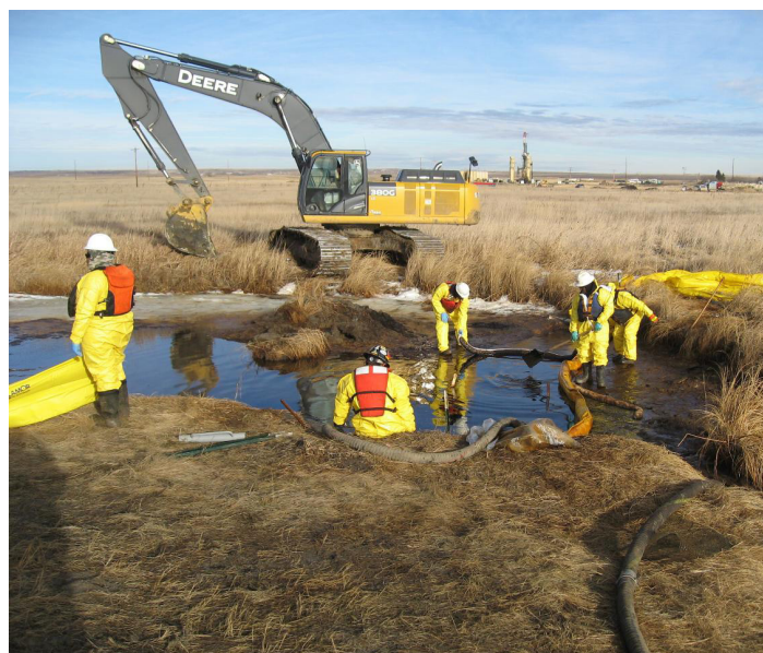
Cleanup crew at the 2015 Blacktail Creek spill, Marmon, North Dakota. This spill was caused by a leaking pipeline that was transporting produced water in the oilfield. Image credit: U.S. Environmental Protection Agency. 24
