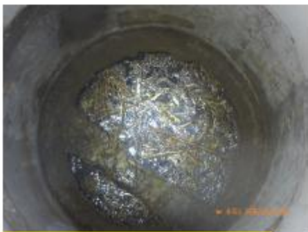
Inlet access port opening – secondary tank
