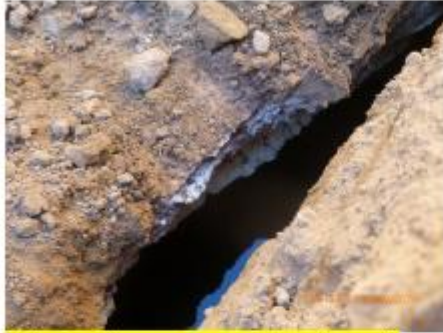
Hole at outlet access port – secondary tank
