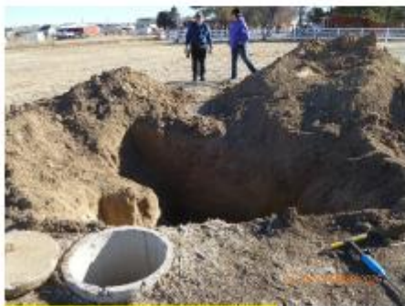
Tank to diverter valve facing east
