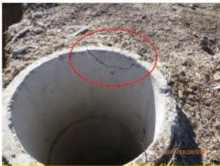
Cracked riser on inlet access port – secondary tank
