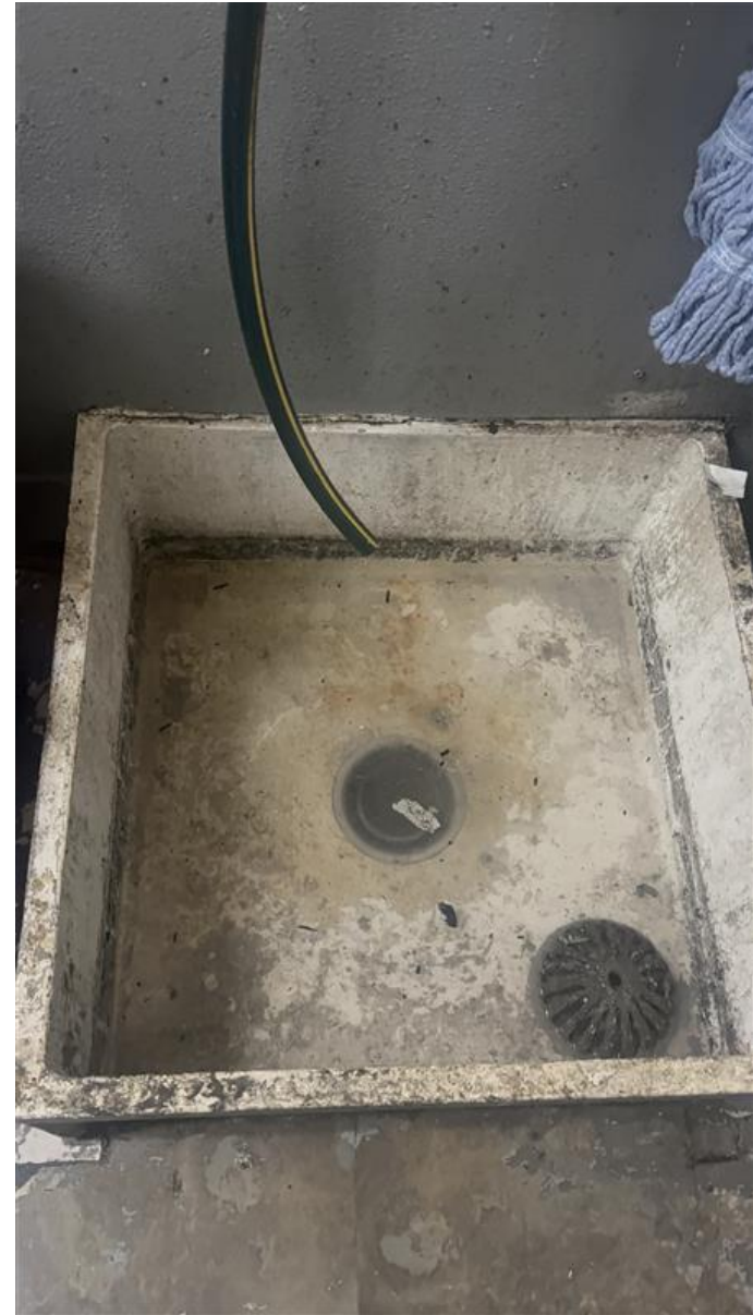
May 1, 2026: Soiled mop sink that is slow to drain and not maintained.
