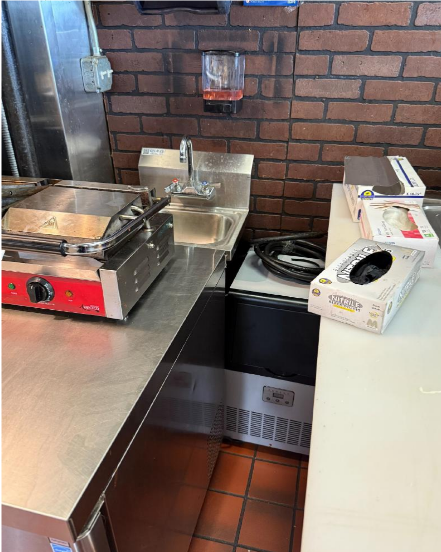
March 13, 2025: Blocked handwashing sink.
