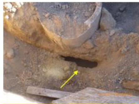
Outlet access port – secondary tank – Damage from the excavator.
