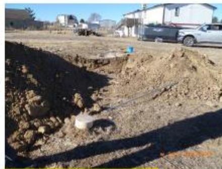
Diverter valve to tank facing west
