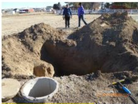
Tank to diverter valve facing east
