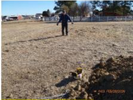
Diverter valve to STA 2 facing east
