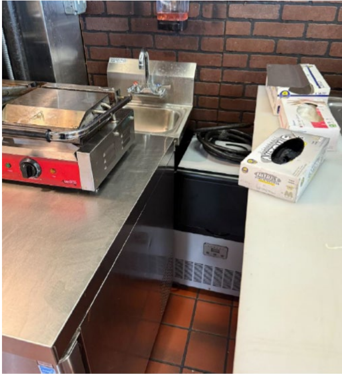
March 13, 2025: Blocked handwashing sink.
