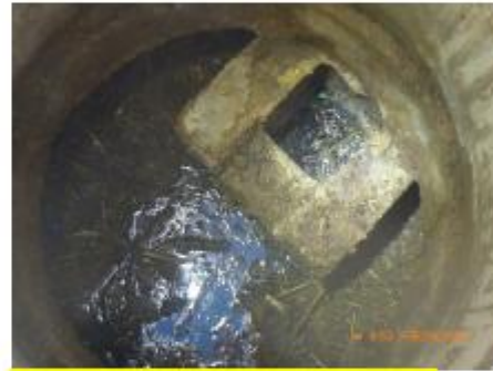
Outlet access port opening – primary tank
