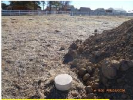
Diverter valve to STA 1 facing southeast
