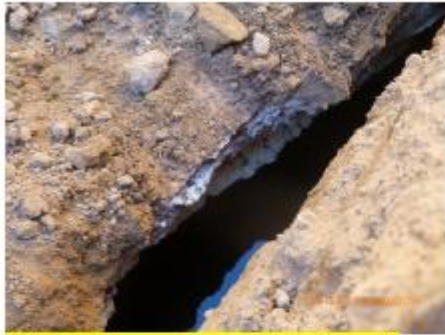
Hole at outlet access port – secondary tank
