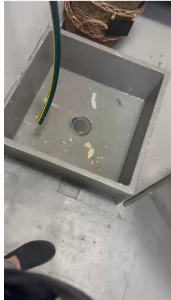
May 13, 2026: Mop sink slow to drain.
