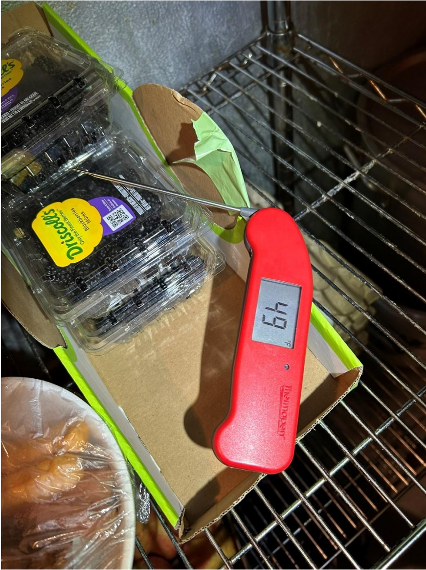
May 13, 2026: Walk-in refrigerator holding at 49F.
