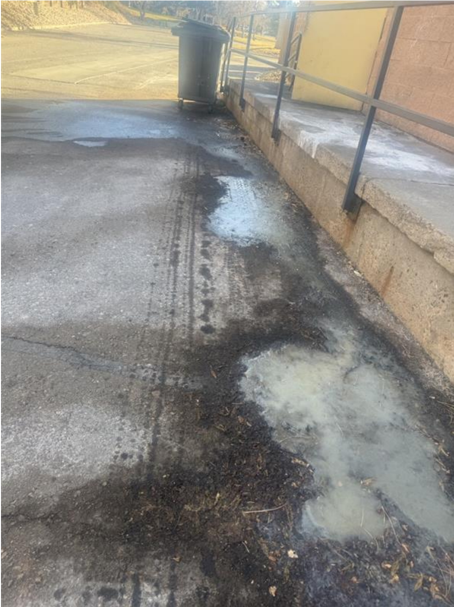
December 18, 2025: Grease spill onto ground outside of business caused by business.
