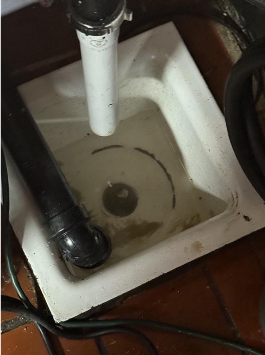
October 28,2025: Clogged floor sink/backup of greywater.
